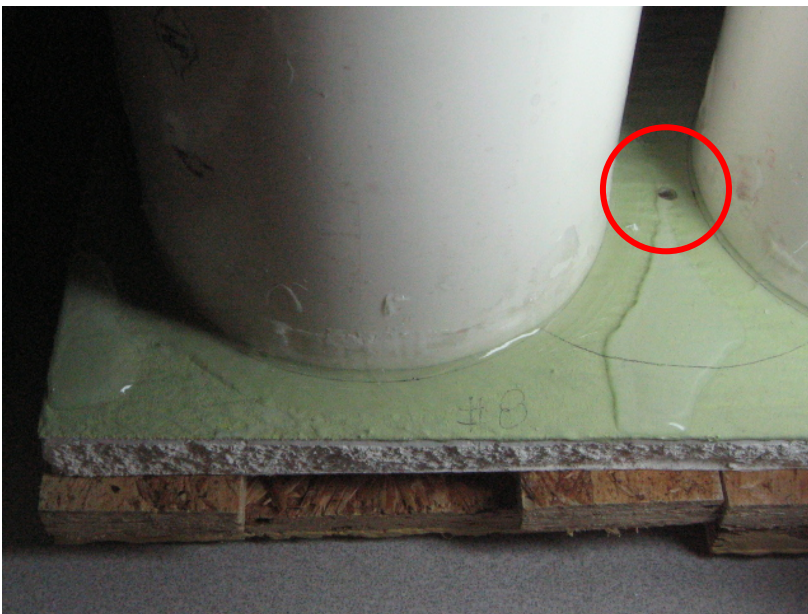
Photo 1. The photo depicts water column testing (the base of two columns are visible) and the presence of water percolating up through the sheathing material during the test (red circle) despite the fact that there was no evidence of water penetration on the back side of the specimens at fastener penetrations. This leads to the conclusion that water by-passed the membrane and traveled within the core of the sheathing.
